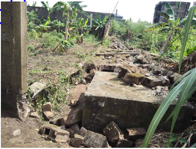
Partially broken fence –Yasa
